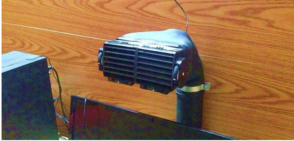
Fig.5: The supply vent
